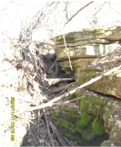
3) 8-foot deep depression with water flowing into bedrock
