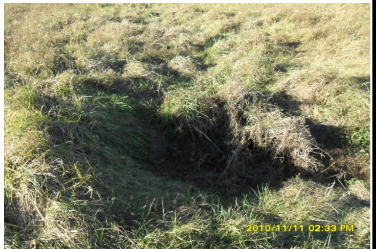
8) 4-foot diameter by 2-foot deep sinkhole
