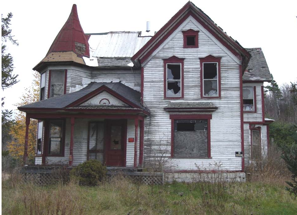
Photograph 4.16. An excellent example of a high style Queen Anne farmhouse on French Creek Road in the Town of Clayton, now abandoned and deteriorating ( PCI 2006 ).
