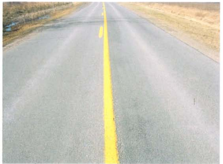
Photograph 2 - County Road 12 on curve
