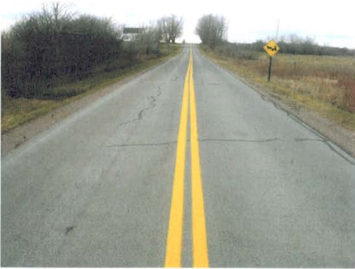
Photograph 19 - DePaulville Road north of Lowe Road
